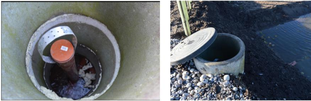
Fig 4. Wells that control the water level in IBZ.
